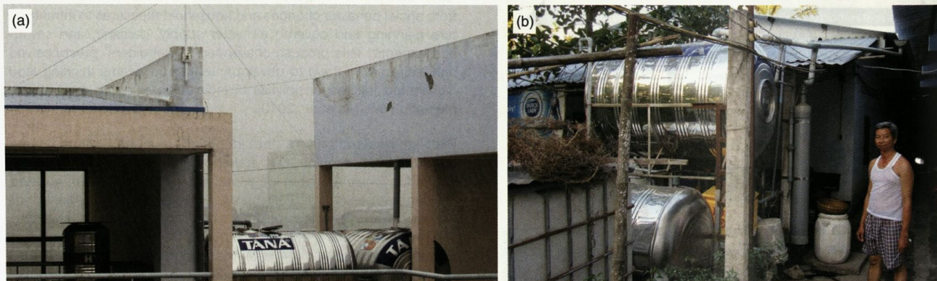
Case Study 14.1 Figure 6 Demonstration of rainwater harvesting systems for safe water supply: One pilot system on Can Tho University campus for research and testing water quality, and one at a peri-urban household in Le Binh ward, Cai Rang District, for reality check.
