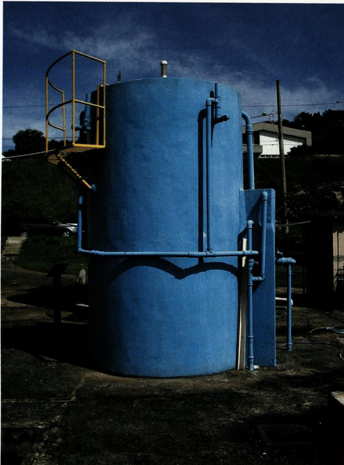
Figure 14.4 A pilot UASB reactor installed in Belo Horizonte, Brazil.
